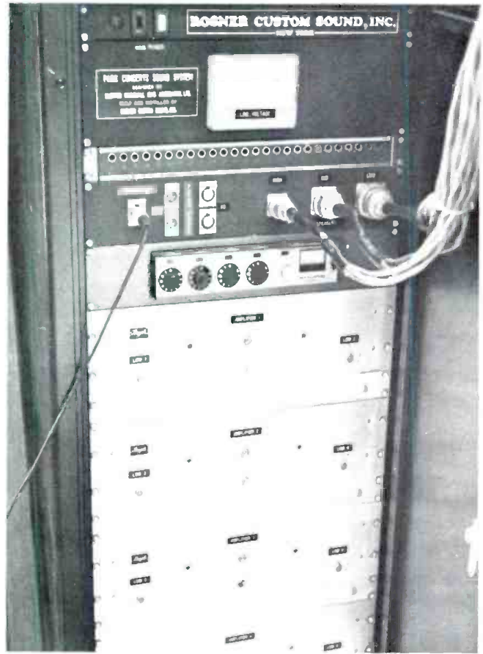
The left of two racks mounted on the speaker tower truck bed has an a.c. line meter, patch and connection panels, a mic mixer, and 4 of the 8 amplifiers in the system.
